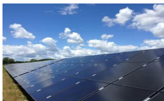
Invenergy's Grand Ridge Energy Center located in LaSalle County, Illinois.
